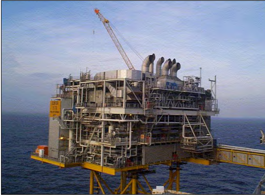
Figure 7.21: Example of a combined cycle power plant installed on an offshore platform on the Norwegian continental shelf [25, ABB, 2000]
